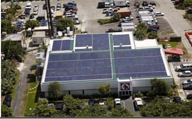
Figure 1, ARI 55.5 KW BIPV Solar System in Ft Lauderdale, FL.
